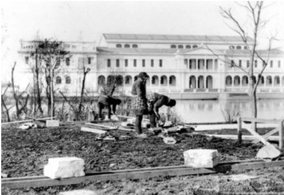
Japanese workers constructing the Hoo-den on the Wooded Island, 1892. Courtesy of the Garden of the Phoenix Foundation.
