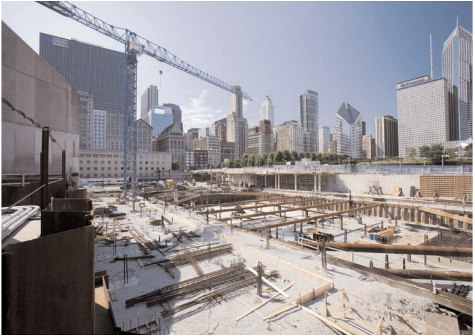
View of the Modern Wing under construction at the corner of Monroe Street and Columbus Drive.
